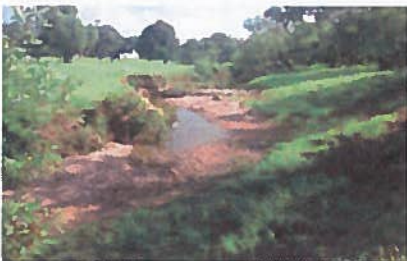
Bank Failure/Channel Widening
