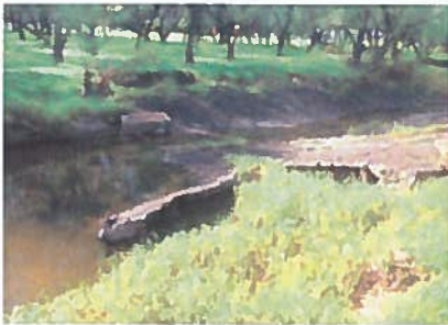
Broken Concrete Channel
