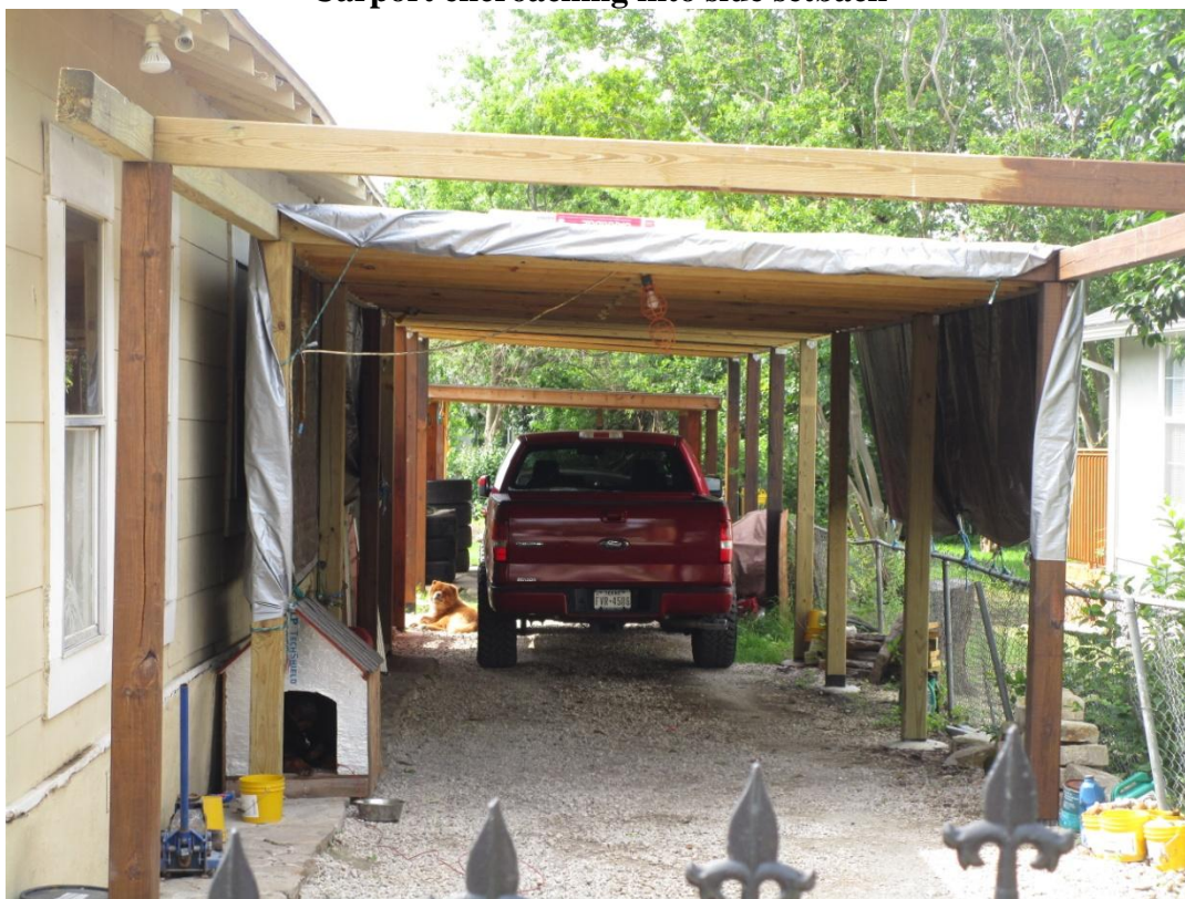
Carport encroaching into side setback
