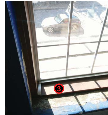
③ EXISTING NON-ORIGINAL WINDOW. CLOSER VIEW FROM INSIDE OF NON-ORIGINAL WOOD SASH
