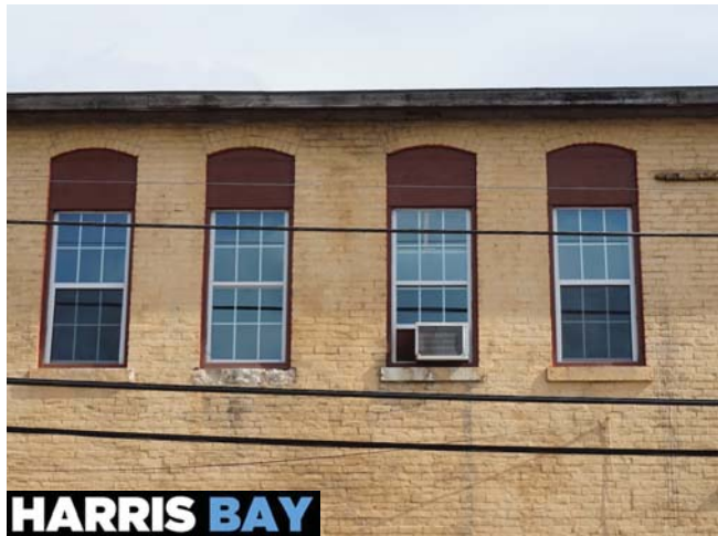
① EXISTING NON-ORIGINAL WINDOW. NON-ORIGINAL WINDOWS ARE INSTALLED THROUGHOUT THE ENTIRE BUILDING
