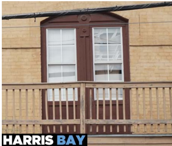
① EXISTING NON-ORIGINAL WINDOW. NON-ORIGINAL WINDOWS ARE INSTALLED THROUGHOUT THE ENTIRE BUILDING
