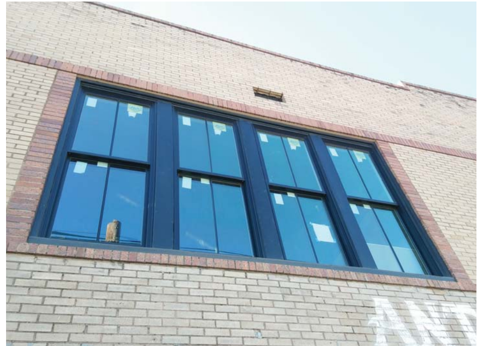
CLOSER VIEW OF INSTALLED, HDRC APPROVED WINDOW AS REFERENCED ON ADJACENT BUILDING "ANTIQUES WAREHOUSE LOFTS"
