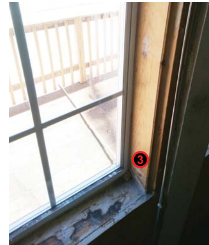
③ EXISTING NON-ORIGINAL WINDOW. CLOSER VIEW FROM INSIDE OF NON-ORIGINAL WOOD SASH
