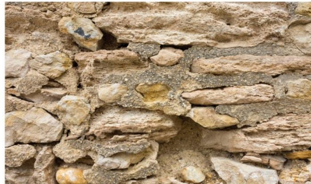
Severe material loss in the zone of rising damp.
