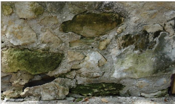
Biological growth that correlates with advanced deterioration at the base of the Long Barrack on the east elevation directly below the canals.
