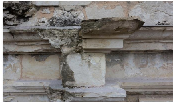
Severe loss of ornamental carved material at the west facade of the Church.
