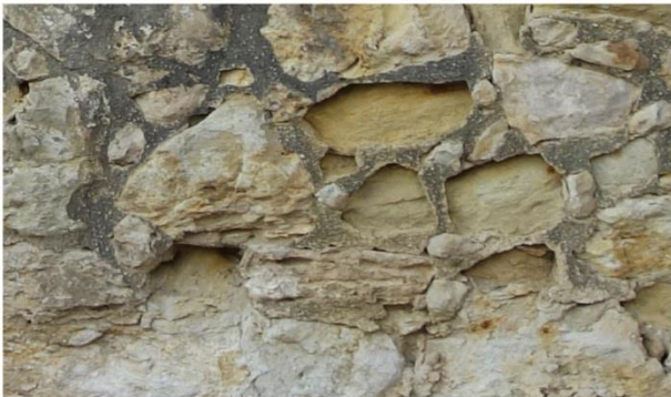
The depth of stone loss due to erosion varies from under 1 inch to 3 inches or more [wall between Long Barrack and Church].
