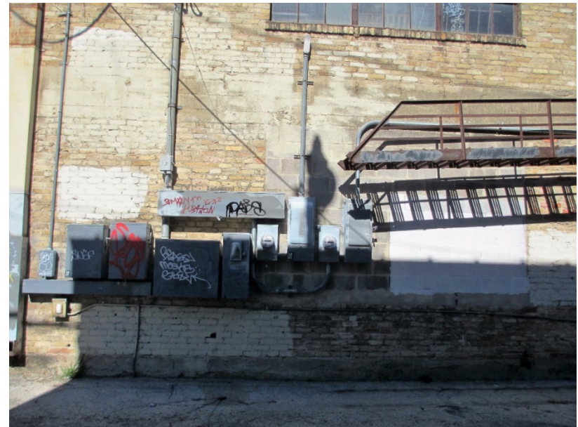
EAST - 1 ST FLOOR AT ELECTRICAL SERVICE
