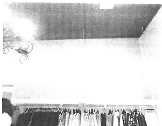
Building 3-Wall moisture and staining
