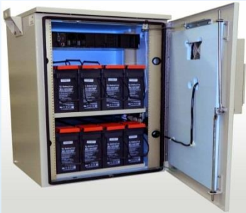
Battery Backup System
