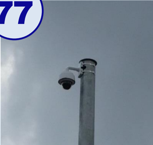
Traffic Monitoring Cameras
