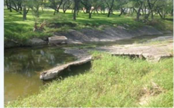
Broken Concrete Channel
