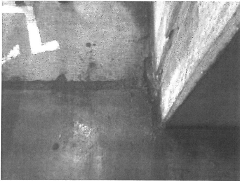
Combination 1" and 2" expansion joints entering the handicap section
