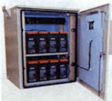
Battery Backup System
