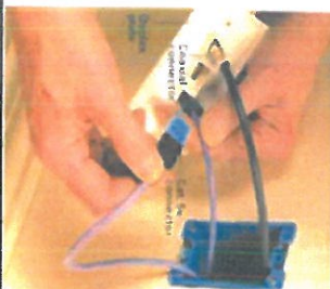
Wall Plate w/ Cat 5e and RG-6
