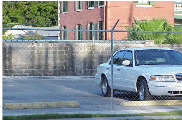
Examples of non-conforming fence material and height (right and below)
