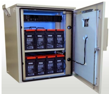
Battery Backup System
