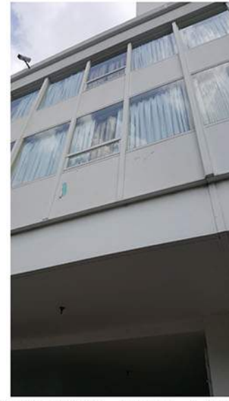
EXISTING BLUE PANEL COVERED & PEELING
