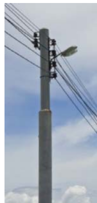
Fig 8.9 Power Lines Attached to Power Pole
