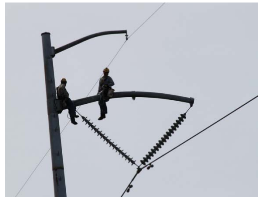
Fig 8.8 Cantilever Arm on Power Pole
