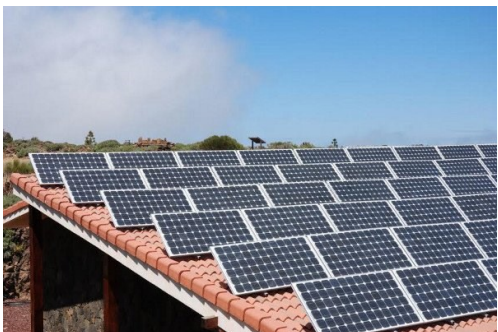
Inappropriate mounting—slope and color
