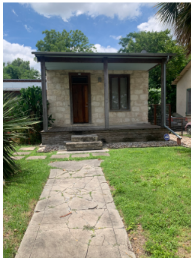
224 Lavaca Broken Concrete
