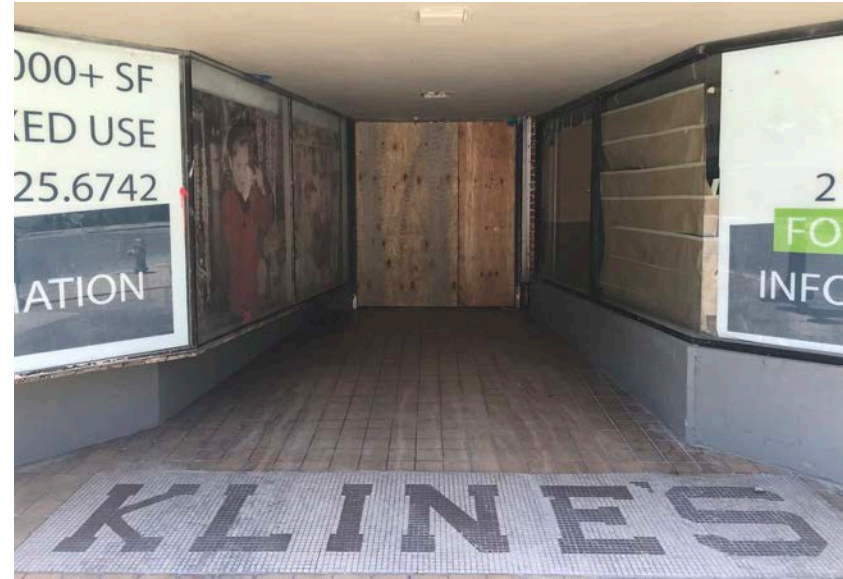
2 EXISTING ENTRY WITH UNEQUAL STOREFRONT CONDITION
