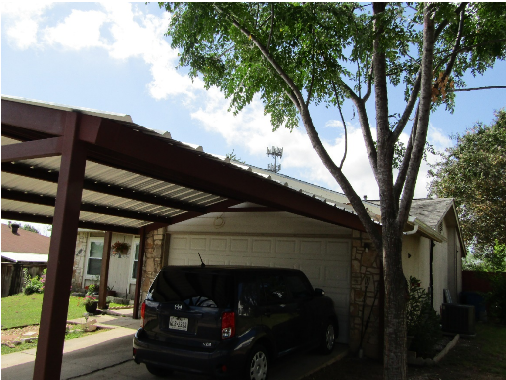
Roof with no Gutters
